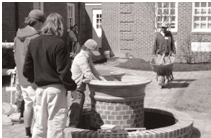
FH subcontractors put finishing touches on the fountain located in the courtyard
